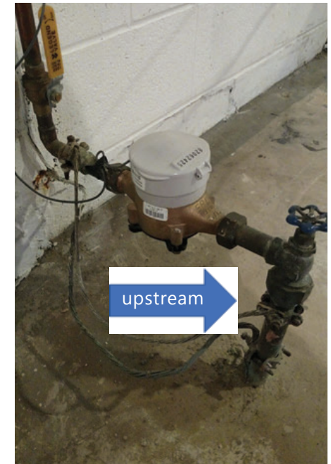
Water meter and service line originating from the floor.
